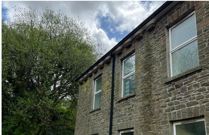
Figure 7. Swift boxes installed on NPTC-owned building in Resolven
